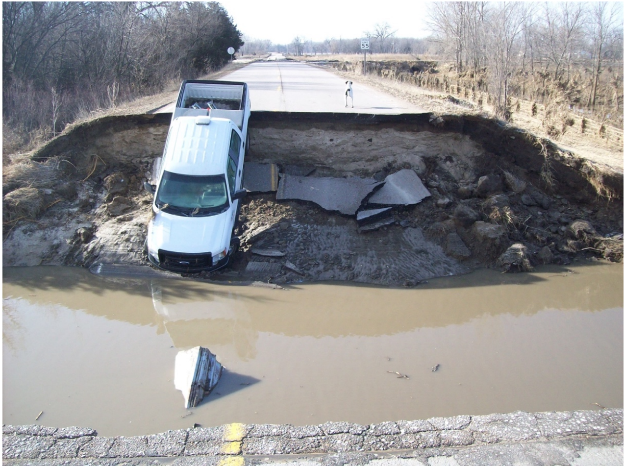
Figure 8 – Photo of Washed Out Road
